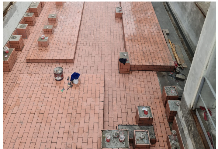
1. Tile Installation - ErgonArmor provided on-site technical support to the contractor during critical surface preparation, tile setting, grouting and detailing stages.
